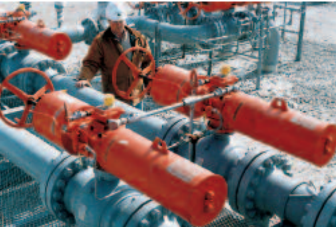
A typical gas pipeline application using the familiar Bettis orange actuators
