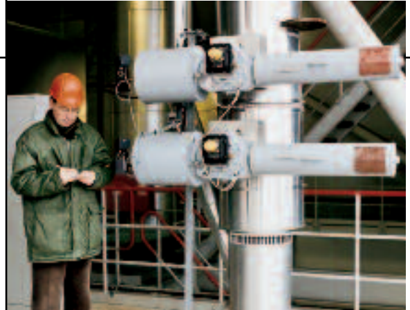
Bettis actuators in service at a major coal gasification plant
